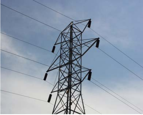
Fig. 5. Sample Steel Tower
